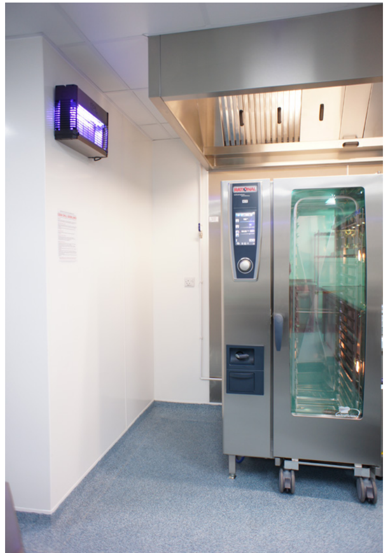
Altro Puraguard in a commercial kitchen
